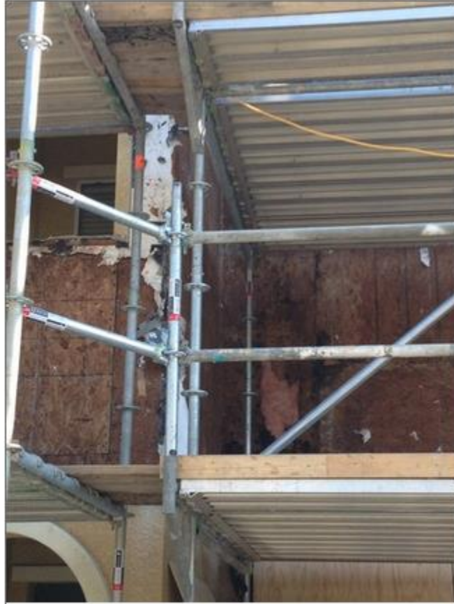
More stucco and rotted wood removed from KB Homes Willowbrook townhomes, getting to the source of water intrusion.
