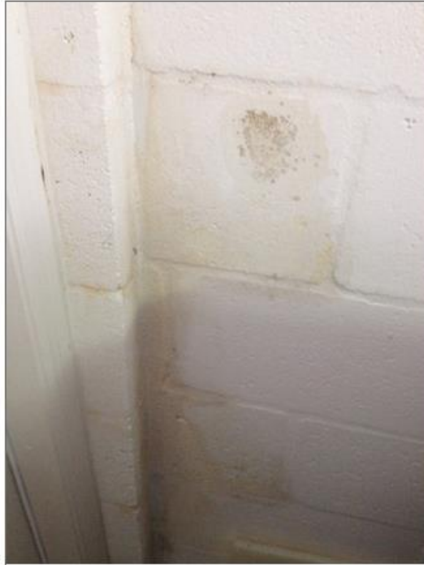
Inside KB Homes garage, mildew on the wall from water intrusion issues.
