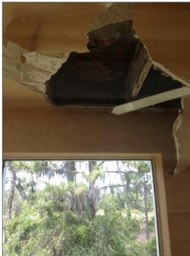
Collapsed balcony ceiling on the exterior of this KB Home
