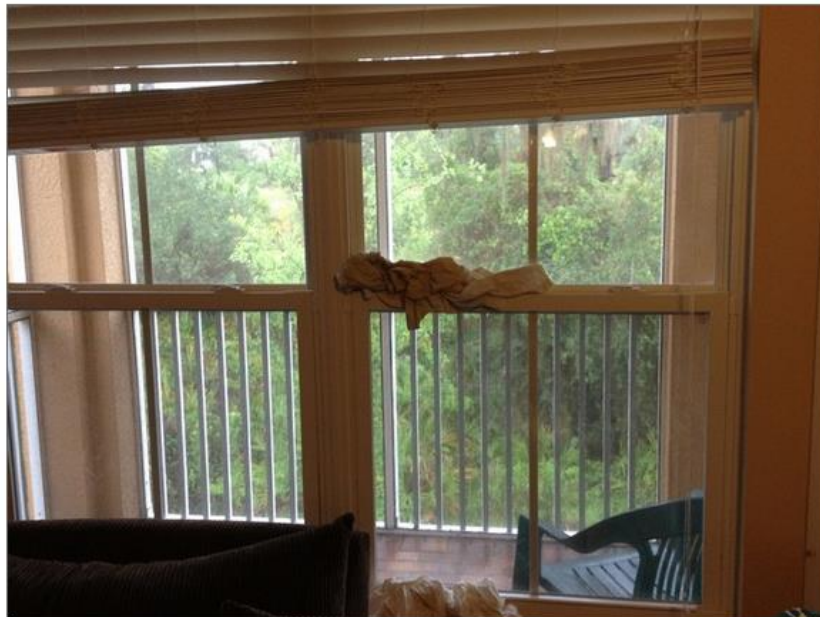
Water damage on the interior of this KB Homes leaves homeowners scrambling for towels and restoration work.
