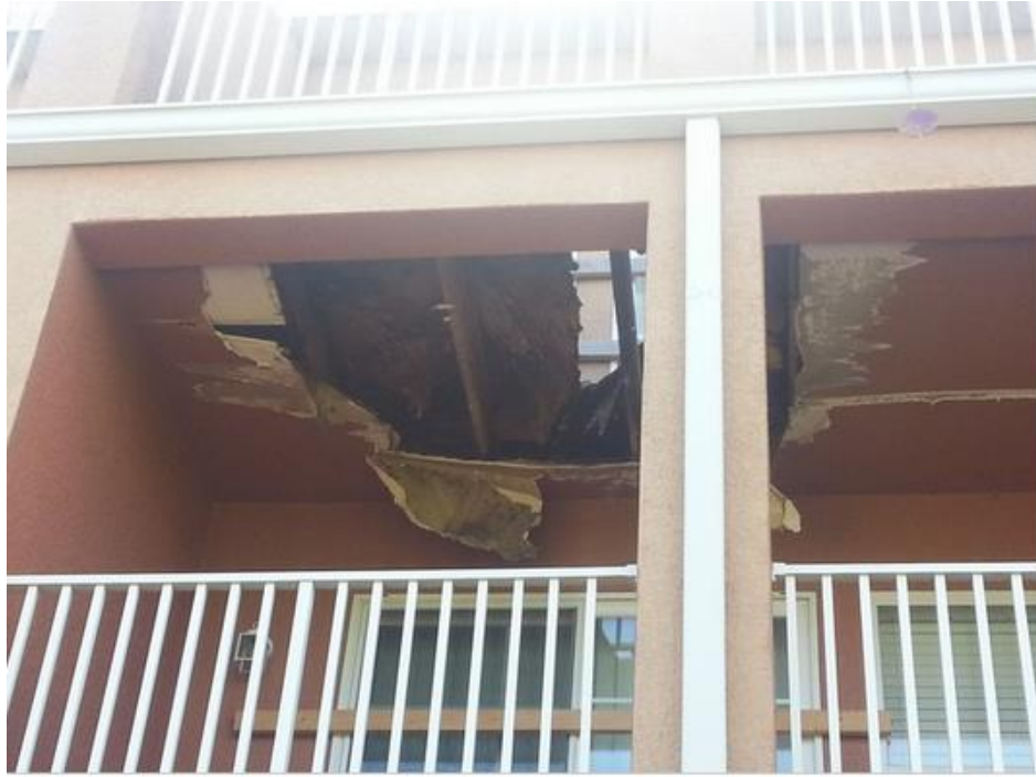
KB Homes Exterior Balcony Failure
