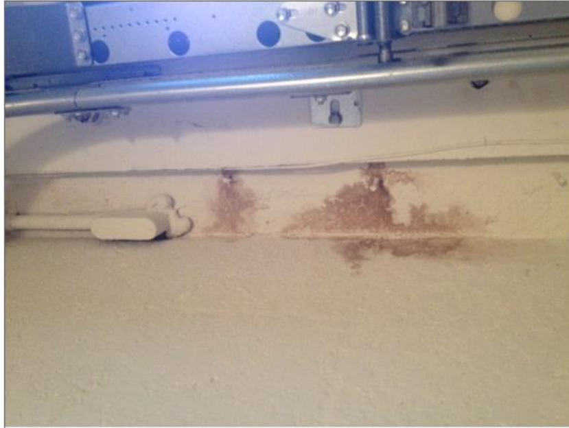
KB Homes water intrusion, mildew and mold in garage from water intrusion on front of building.
