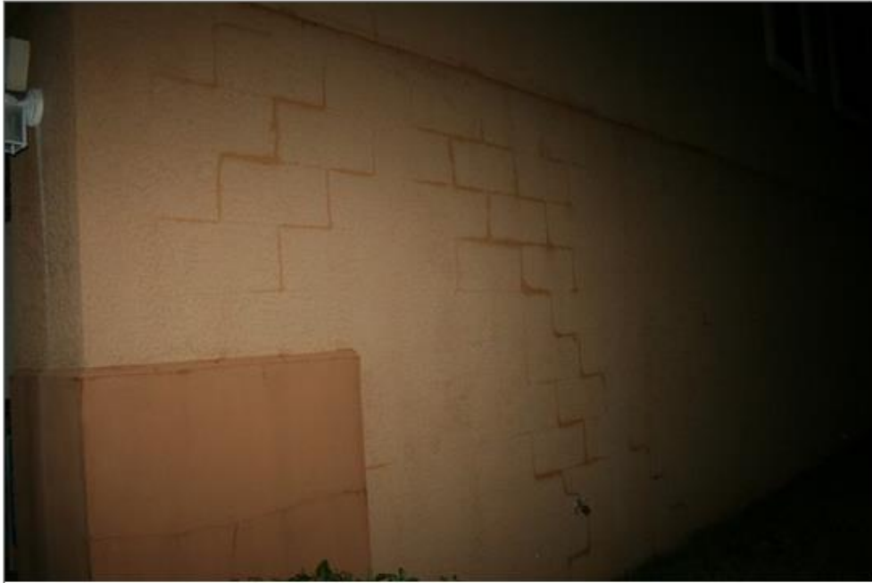
Water Intrusion on Exterior of KB Homes
